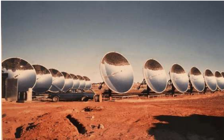
Gambar 6.10 Instalasi Australia National University di White Cliffs [61]
