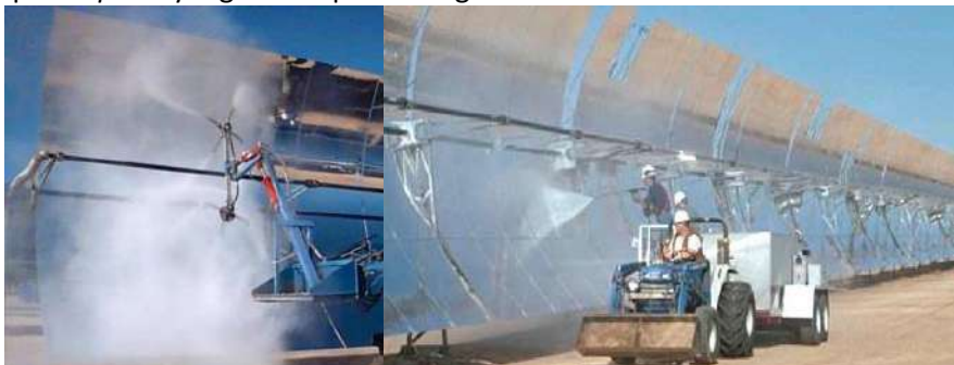
Gambar 4.18 Metode pembersihan cermin di plant CSP, a) robotic arm , b) manual [48]
